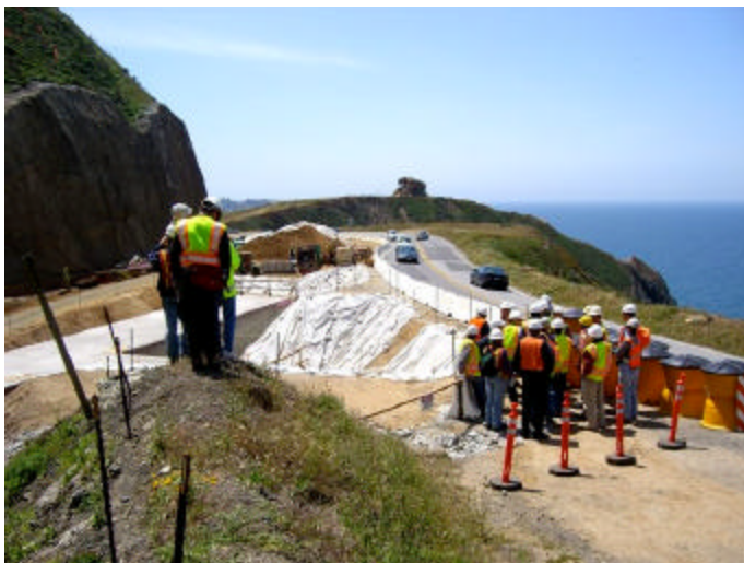
Drainage Culvert at South Entrance to Tunnels; View to South; New Road Bed to Left
