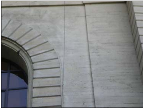
Figure 3 Tension cracks on the side of the Berkeley Memorial Stadium north entrance.
