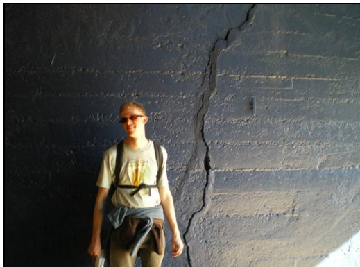
Figure 4 Large fracture in the wall at the north Berkeley Memorial Stadium entrance below the bleachers.
