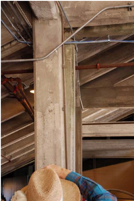
Figure 6 Offset along pillars underneath Berkeley Memorial Stadium.
